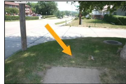
Photo C-5: Sidewalk Abruptly Ends
